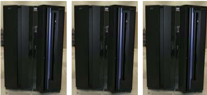
Data Center Heron
