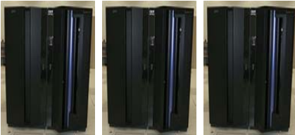
Data Center St. Laurent
